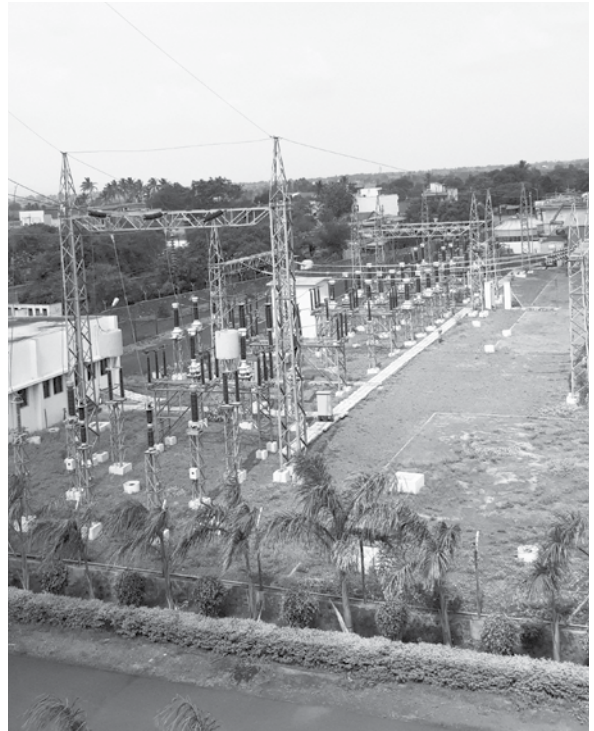
Co-Generation Power Project set up by Pravara Renewable Energy
