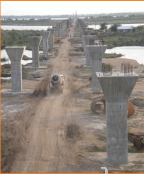
Rajahmundry Godavari Bridge Limited (RGBL)
